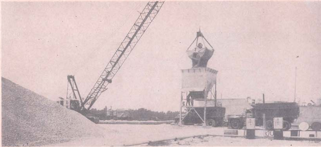
Loading shells at the Harvey Canal yard of Ayers Materials Company into trucks for delivery for use on roadways, parking areas and drilling sites. Shells are also loaded for barge or rail shipment.
