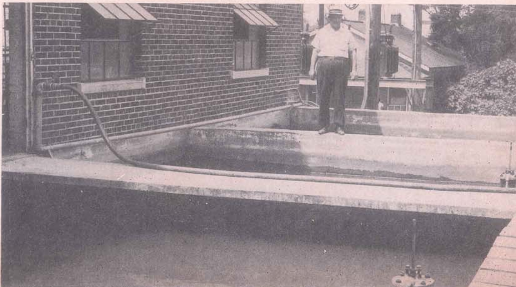
Superintendent Eugene Gehring of the Greटना Water Department shows the Review photographer the four filter basins in which new vitrified clay bottoms have recently been installed at a cost of $17,000.
