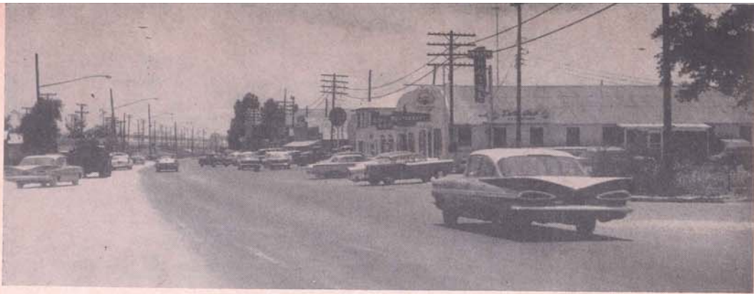
A view of the West Bank Highway's 24 foot widening program — showing the completed work at the Port Sulphur main section of town.
