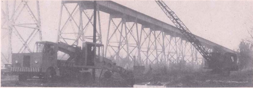
Showing the excavation of a Jefferson Parish drainage canal with Gradall and Drag Line, part of the detail work of improving and modernizing the East Bank drainage system to more satisfactorily serve a rapidly expanding population.
