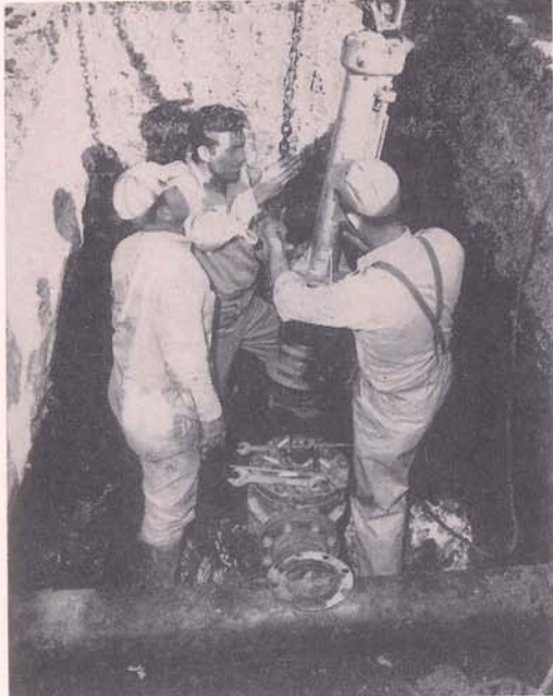
The expert workmen of the Louisiana Gas Service Company of Harvey extend a six inch, high pressure gas main to insure an abundant supply of natural gas for industries along the Harvey Canal.
