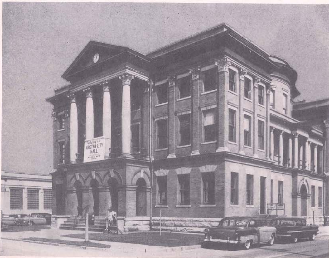
The historic Old Court House of Gretna, now being remodeled and renovated for its new identity in the near future as the Gretna City Hall.
