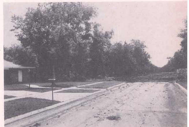
A new section of paving with subsurface drainage in Gretna—a part of the huge $790,000 city wide street improvement program now going on and scheduled to be completed by the end of 1961.
