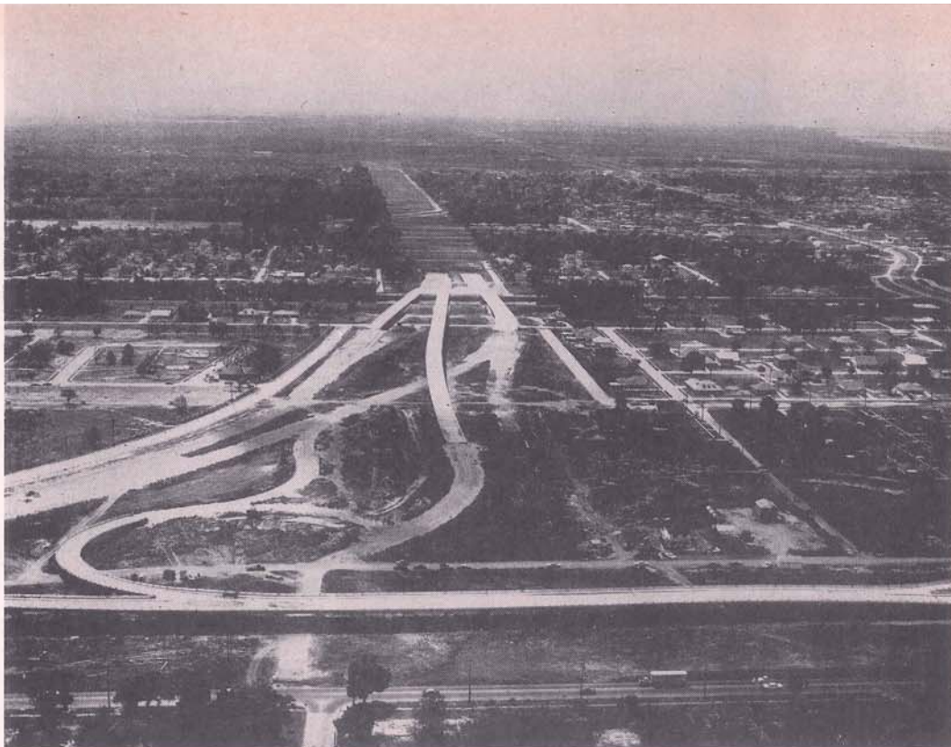
The Pontchartrain Interchange now under construction looking west into Jefferson Parish, showing the right of way cleared to Causeway Boulevard.
