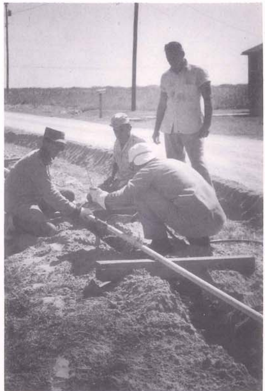
Installing the natural gas distribution system on one of Grand Isle lanes.
