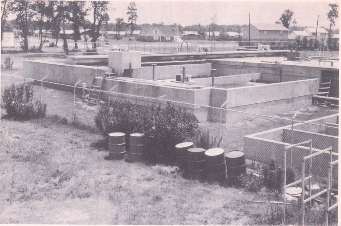
The West Bank completed sewerage treatment plant at Terrytown—part of the construction program that will bring modern sanitary sewerage systems to the populated portions of Jefferson's entire unincorporated areas on both East and West banks.
