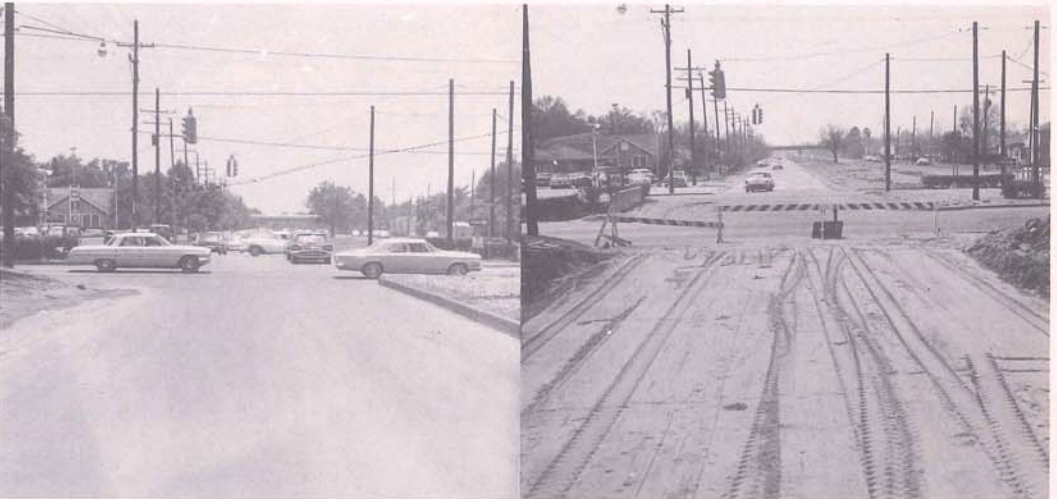
Road construction on Bonabel Boulevard in Metairie. Right shows how after top soil was removed tons of river sand were placed as a base and picture left shows same boulevard after the pavement was laid.
