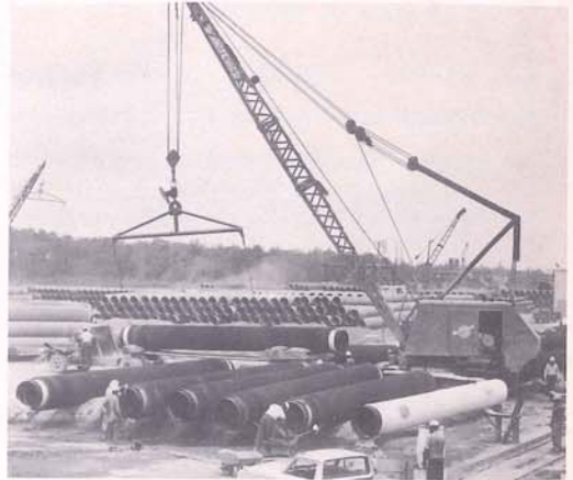
A section of the storage yard at the H. C. PRICE Company's Coating Division at Harvey in Jefferson Parish. This plant has been awarded contracts for covering 1,510,000 feet of pipe into its Somastic corrosion protecting coating. This pipe will be laid in the Gulf of Mexico and the South Louisiana marshes.
