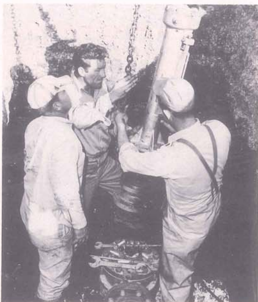
In keeping with the growth in Jefferson Parish, Louisiana Gas Service Company installs a valve while tying in a new 6" gas main extension to one of their existing high pressure mains.
