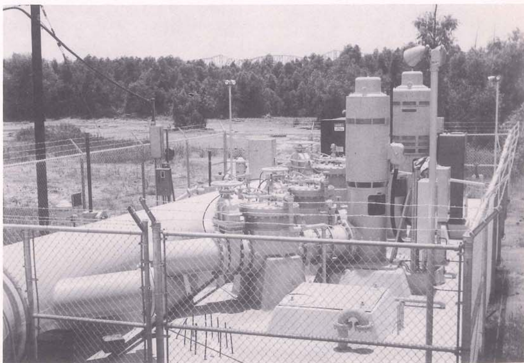
The new 40 million gallon per day Raw Water Intake Line and Pumping Station at the batture of the Mississippi River at East Jefferson Water Works District No. 1 completed early in 1964 at a cost of $545,000. This is part of the never ceasing construction program of the Jefferson Water Department financed out of revenue to keep pace with the population increase and the industrial, commercial and residential expansion of Jefferson Parish.
