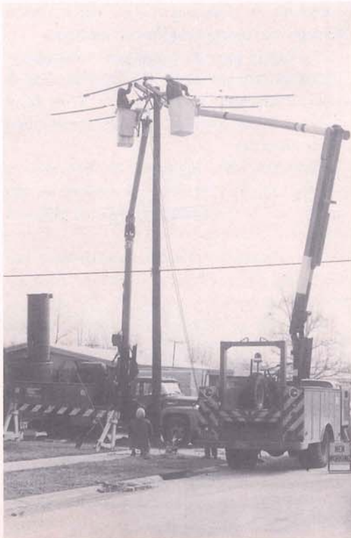
Relocating a power line on East Bank to permit installation of a lift station in the present sewerage construction program.
