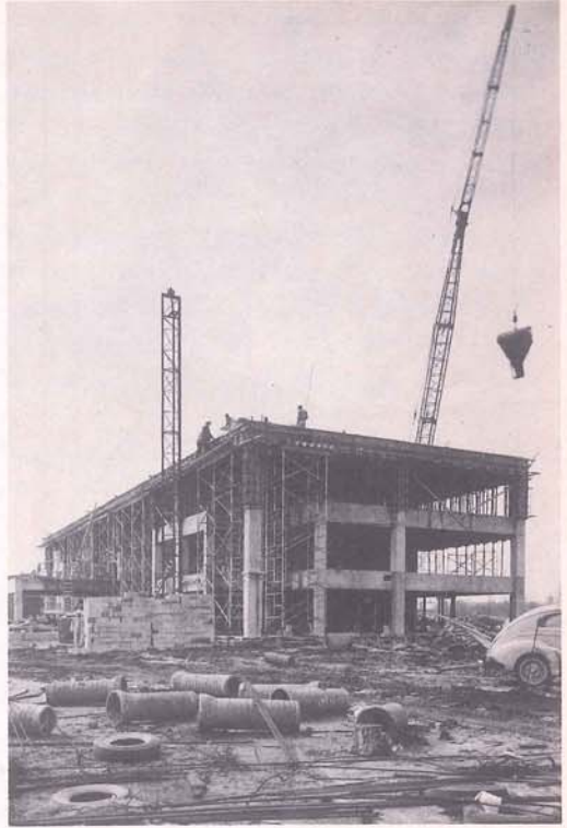
The new incinerator under construction in Garbage District No. 1 (East Bank) right behind the present facility. When completed the present incinerator will be remodeled and put back in operation.
