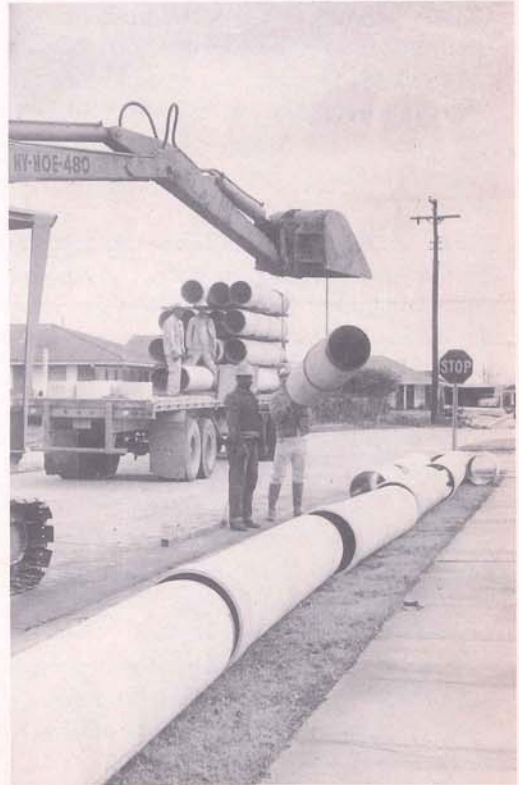
Installing 18 inch epoxy lined sewer pipe at Kewanee and Olympic in the current parish wide sewerage construction program.
