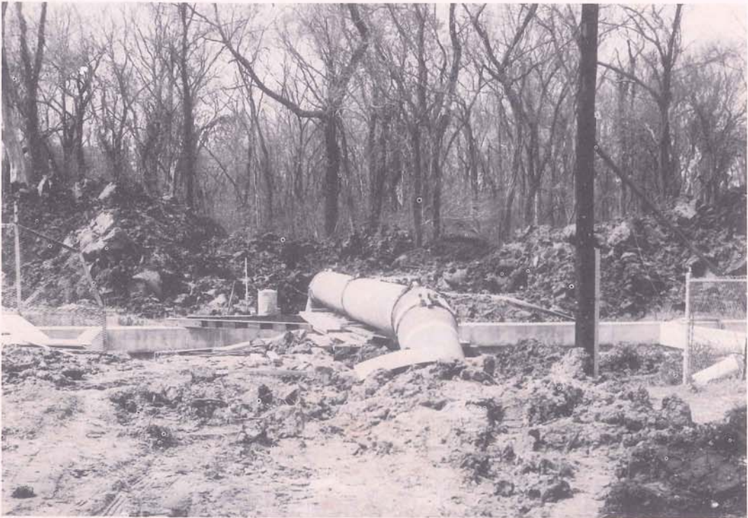
The placing of a 24 inch water main across Soniat Canal adjacent to the Harahan Playground. This is a segment of the 1964 new construction program of the Jefferson Parish Water Department — to better serve a growing and expanding parish.
