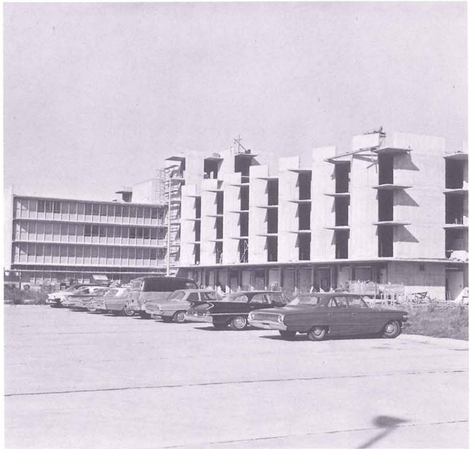
Expansion and renovation program at West Jefferson General Hospital will add 100 beds to existing 160-bed facility at a cost of $2.5 million. Picture shows 52 per cent completion reached on November 1, 1966.
