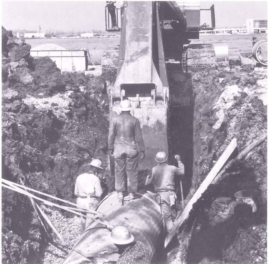
Huge 42 inch water main is installed along Duncan Canal in Kenner as work progresses on East Jefferson Master Water Plan.
