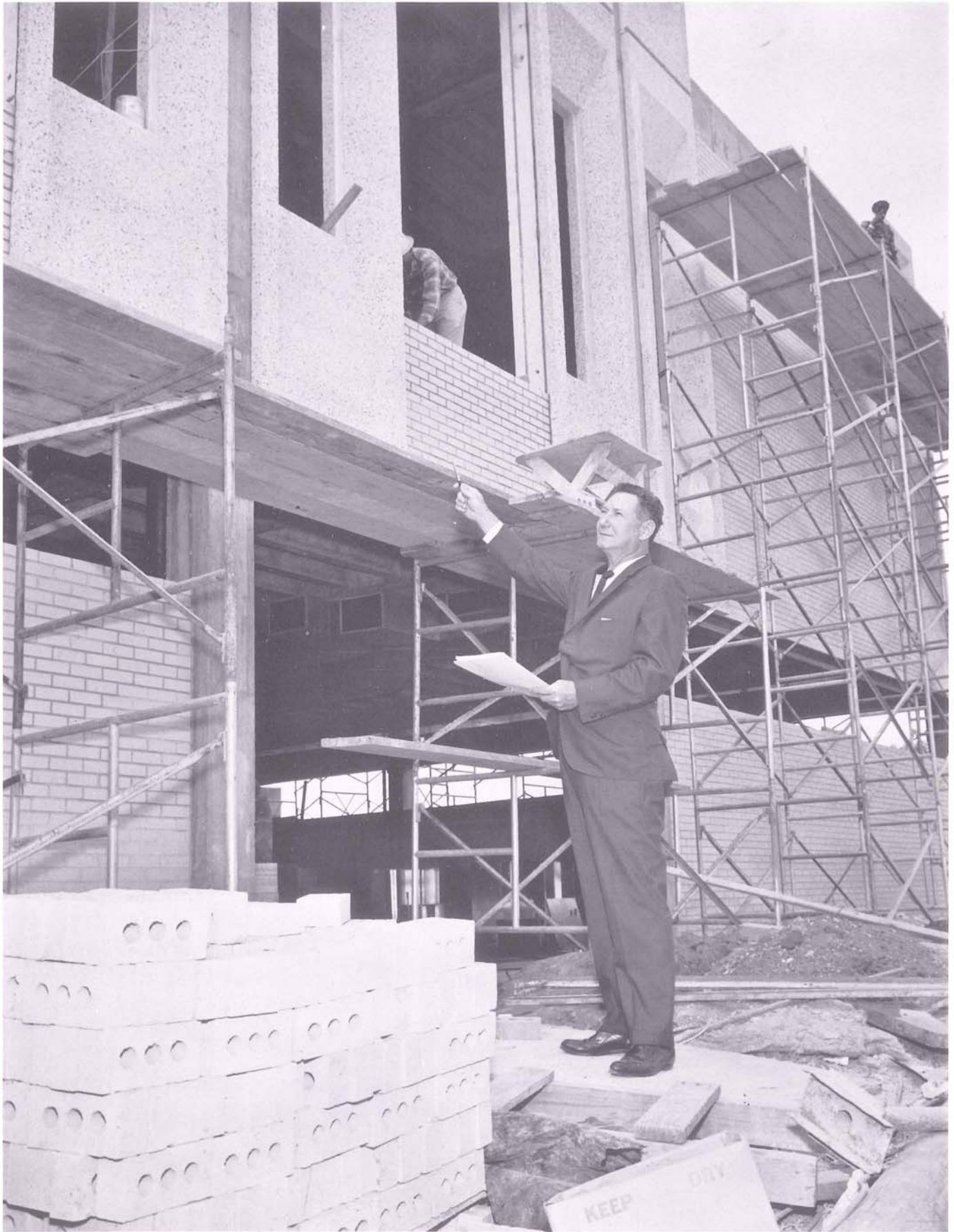
Clerk of Court William M. Justice, Jr., checks construction progress of the new Jefferson Parish court building scheduled for completion in June 1968. The $1,132,350 two-story building will house the civil and criminal court section of the clerk of court's office on the first floor plus a juvenile court complex and district attorney's offices. Six new courtrooms are planned for the second floor.
