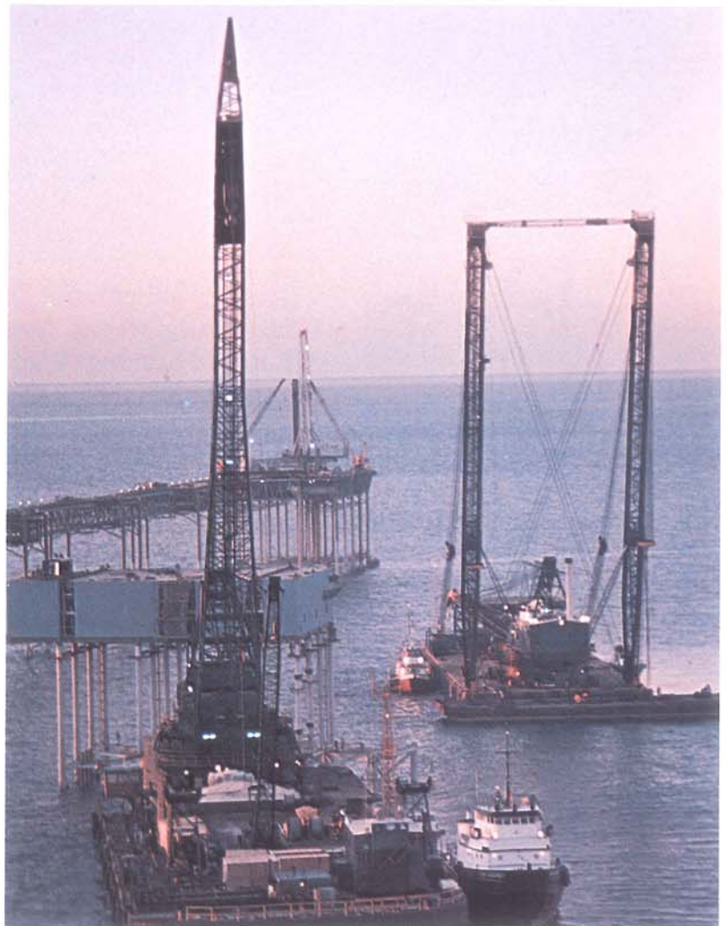
Derrick barges lift record 800 tons in construction of industry's newest major sulphur mine at Caminada, six miles off Jefferson's Gulf Coast. Caminada and Grand Isle (both in Jefferson), the world's only off-shore mines, are operated by world's largest sulphur producer.
