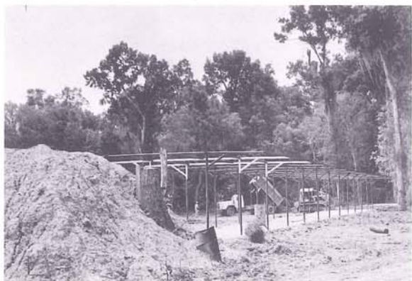
Under construction on Barataria blvd., near Estelle on the west bank is the sprawling new sheriff's firing range with separate facilities for pistol and rifle target practice.
